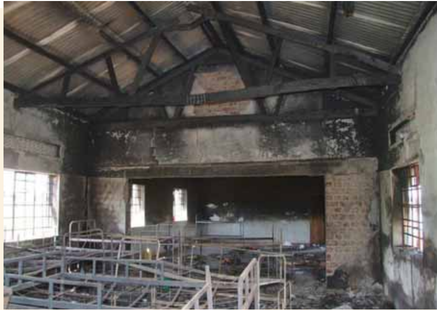
Inside the Boys Dormitory after the fire
